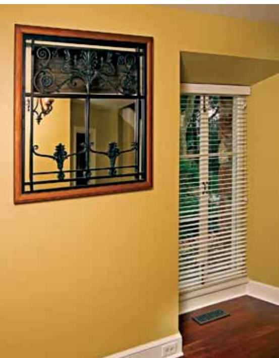
ABOVE: Air-return grilles are incorporated into the home's décor. TOP: The kitchen and dining room were in such poor shape that they had to be gutted, allowing the Neiblums to run ductwork under the floors.
